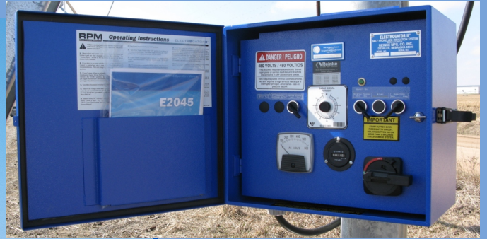
Main Control Panel
